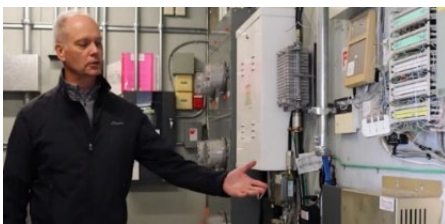
Figure 3. A condo owner in Saanich, BC shows the upgraded electrical infrastructure and panels that were part of the EV ready retrofit in his building. Source: District of Saanich.
